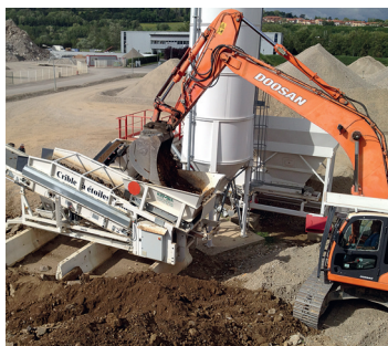
Installation de chaulage.
